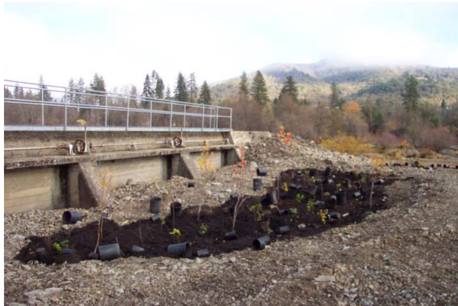
Figure 4-5: Example of an excavated area for planting backfilled with soil to promote plant growth.
