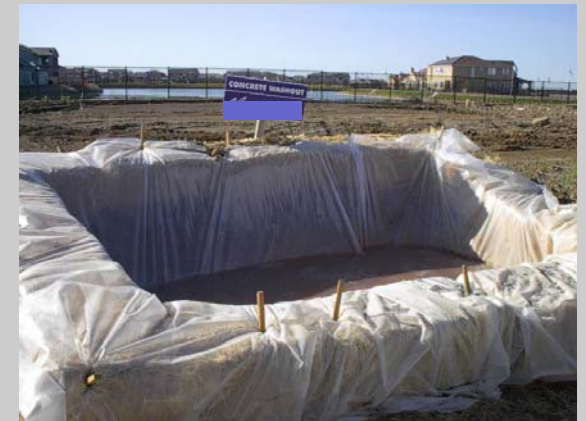
An example of a properly designed concrete washout. Washouts can be scaled down for use on smaller projects.
