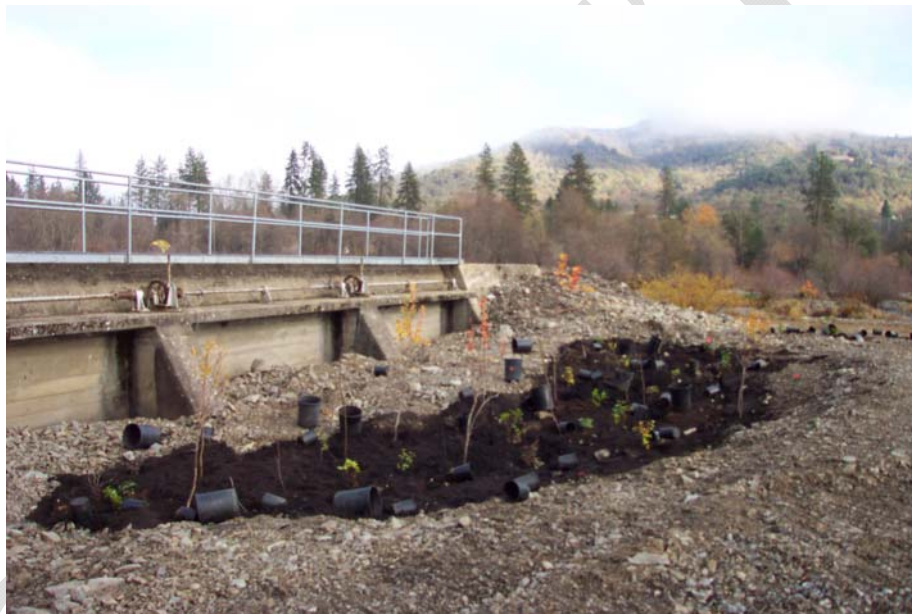
Figure 3-3: An example of a irregular planting bowl and soils brought in for native plants as part of a restoration project.
