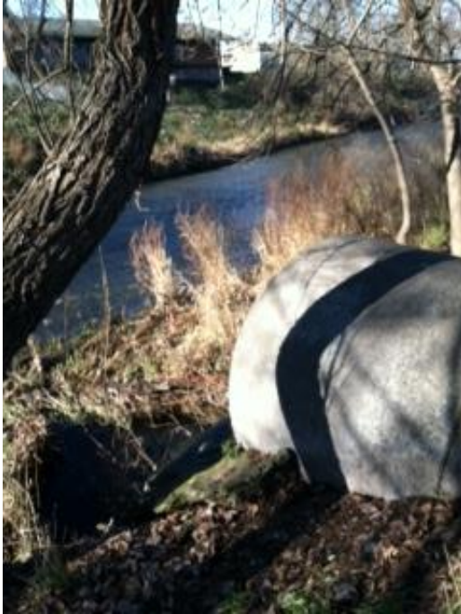
Stormwater cement pipe outfall.
